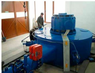
HPP Zla Reka (Bulgaria) Turbine type: Pelton VS4 Net head: 83 m Discharge: 0,4 m 3 /s Speed: 600 rpm Nominal output: 0,290 MW
