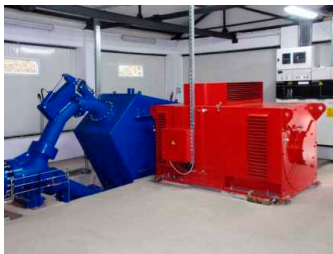
HPP Balea (Romania) Turbine type: Pelton HS2 Net head: 385 m Discharge: 0,53 m 3 /s Speed: 1000 rpm Nominal output: 1,8 MW
