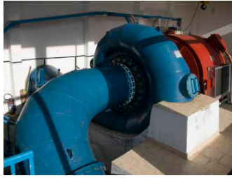
HPP Katunski (Bulgaria) Turbine type: Francis HS Net head: 97 m Discharge: 4,0 m 3 /s Speed: 750 rpm Nominal output: 3,408 MW
