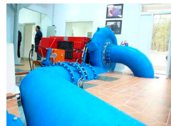
HPP Radac (Kosovo) Turbine type: Francis HS Net head: 34 m Discharge: 1,5 m 3 /s Speed: 1000 rpm Nominal output: 0,445 MW
