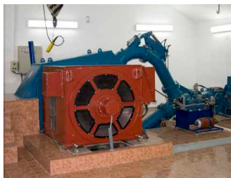
HPP Vodemil (Bulgaria) Turbine type: Pelton HS2 Net head: 104 m Discharge: 0,4 m 3 /s Speed: 600 rpm Nominal output: 0,36 MW
