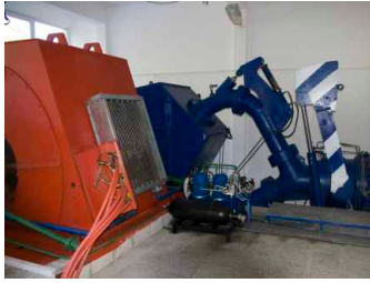
HPP Retije 3 (Bulgaria) Turbine type: Pelton HS2 Net head: 525 m Discharge: 1,1 m 3 /s Speed: 750 rpm Nominal output: 5,1 MW
