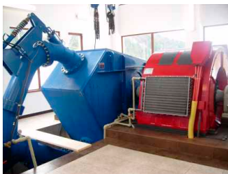
HPP Dzherman (Bulgaria) Turbine type: Pelton HS2 Net head: 259 m Discharge: 1,18 m 3 /s Speed: 600 rpm Nominal output: 2,7 MW
